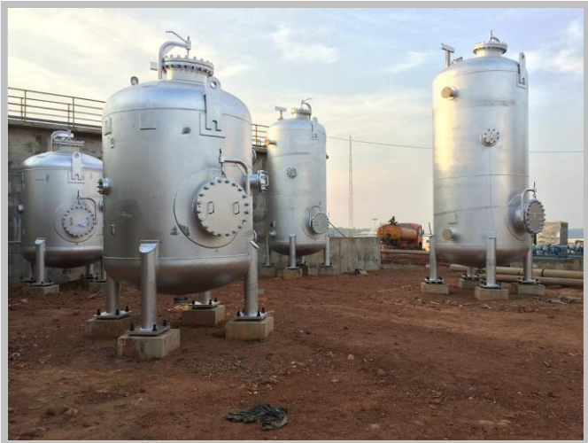
Pressure Sand Filter & Activated Carbon Filter
